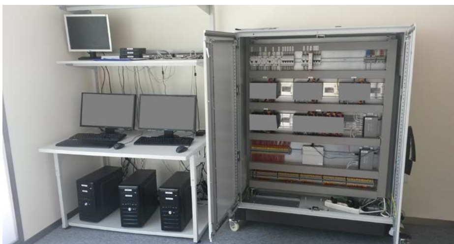
Figure 3: SCADA real equipment
