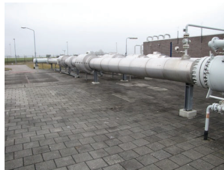
Figure 5: Example of a designed bearing support that is not designed for earthquakes ("one foot support")
