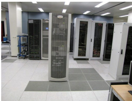
Figure 6: Raised floors and cabinets in control room on a raised floor.
